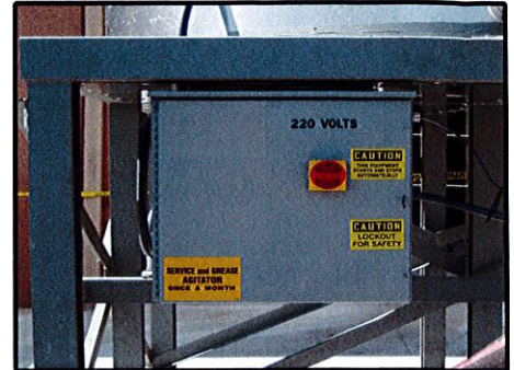
Electrical control panel and agitator timer is enclosed within a single weatherproof NEMA 3R enclosure.
