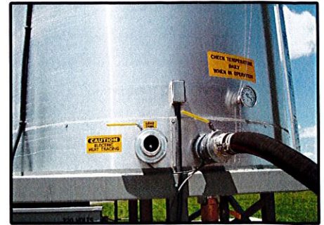
Heated & Insulated ball valves at the base of tank gravity feed emulsion to the Total Patcher.
